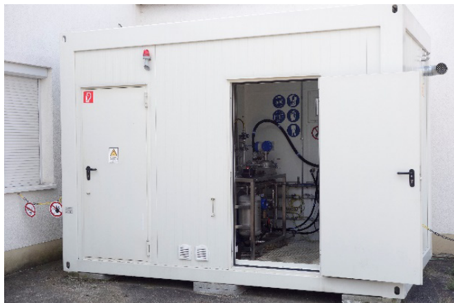
Mobile filtration container.
