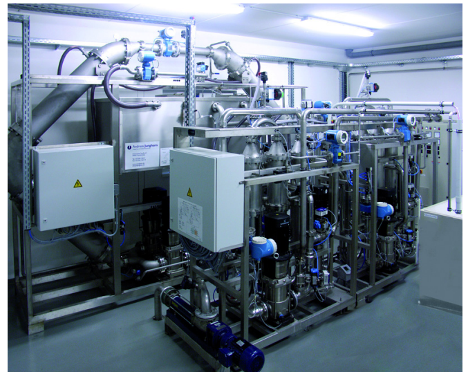
Nanofiltration plant built by company Andreas Junghans.
